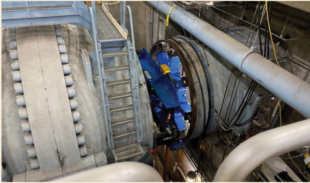
The primary valve at the Rocky Mountain Hydroelectric Plant with in-place machining equipment (blue/yellow) is visible on the right. Valve scale is 11 ft. I.D. (Photo courtesy of Voith and Oglethorpe Power.)
