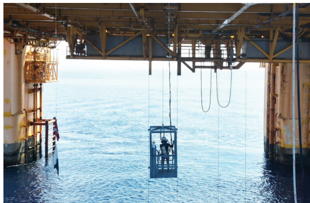
Phoenix International divers finished underwater inspection of almost 600 welds at the Thunderhawk platform in the Gulf of Mexico.
