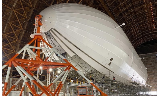
Above is an airship docked to a mooring mast. Numerous airship parts and components as well as the mooring mast itself were built. Everything was welded from 12-in. I-beams to 0.035-in.-wall titanium tubes.
