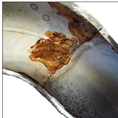
Internal weld geometry can accelerate corrosion-erosion even when a weld meets inspection requirements.
