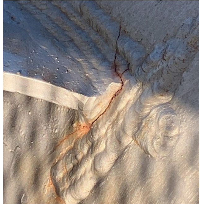
Fig. 1 — In-service crack on a welded repair.
