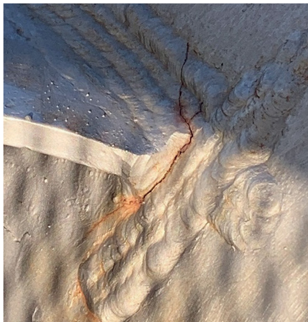
Fig. 1 — In-service crack on a welded repair.
