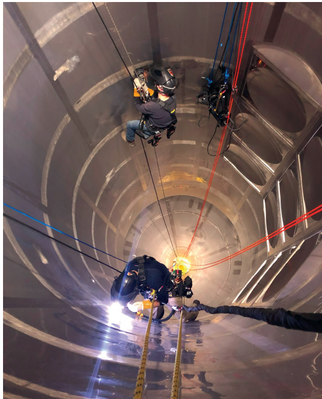
Inspection and weld repairs using rope access inside a vessel. (Photo courtesy of Rigging International Group.)
