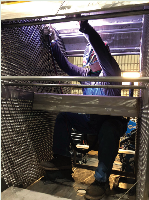
Fig. 3 — Observing welders perform tubesheet gas tungsten arc welding (GTAW) in the fabrication of a feedwater heater.
